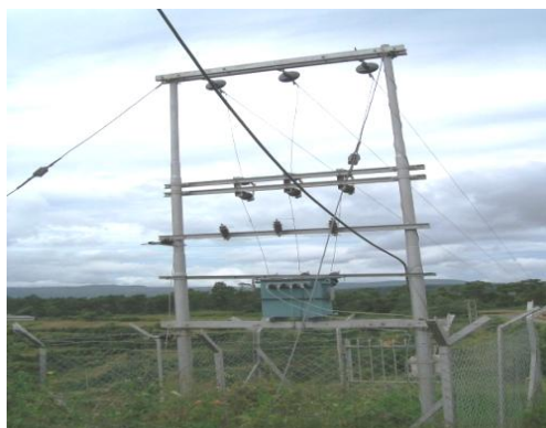
RGGVY Transformer Installed in Tasku Village in Ri Bhoi District
