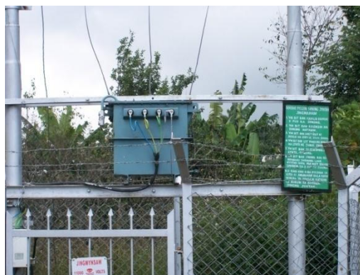
RGGVY Transformer in Jyntah Village of East Khasi Hills District
